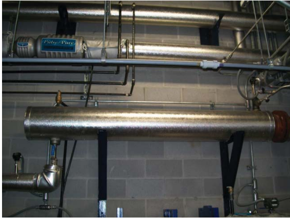
Figure 10: Shell and tube heat exchanger for rejecting heat to the cooling water.
