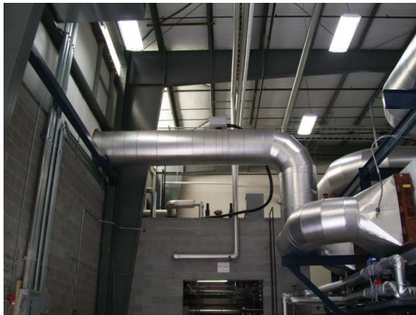
Figure 8: Analyzer location in outlet duct work to monitor downstream emissions.
