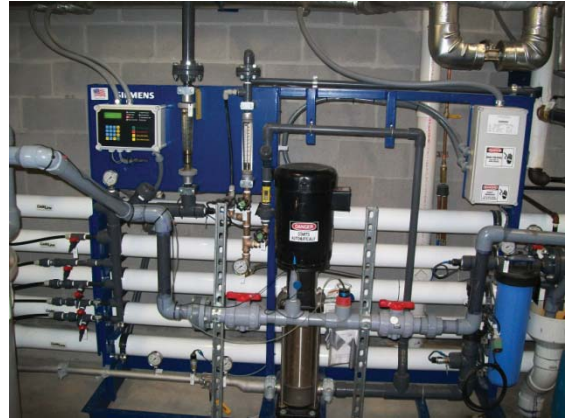
Figure 11: Reverse osmosis water skid.
