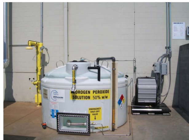
Figure 7: Hydrogen peroxide storage tank with pumping station on left.
