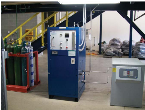
Figure 6: Ozone generator with chiller on right and oxygen bottles on left.
