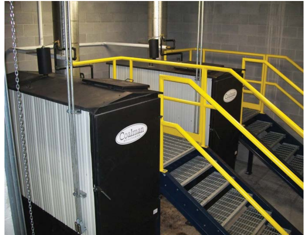
Figure 5: Two coal-fired burners for demonstrating NO x & SO x reductions.
