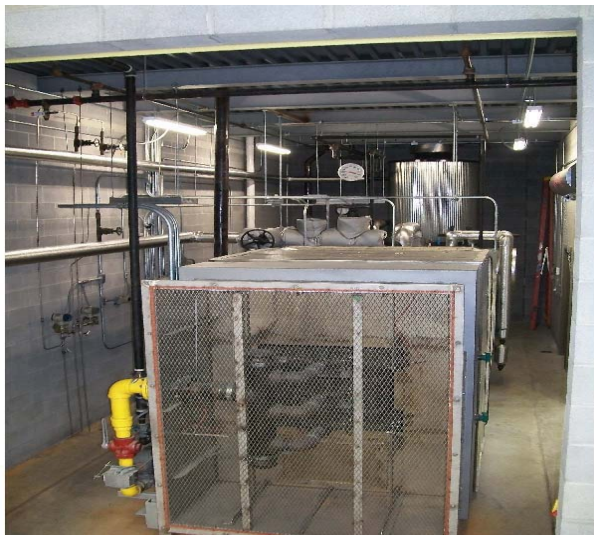
Figure 2: Natural gas burner with wasteheat boiler in the back.
