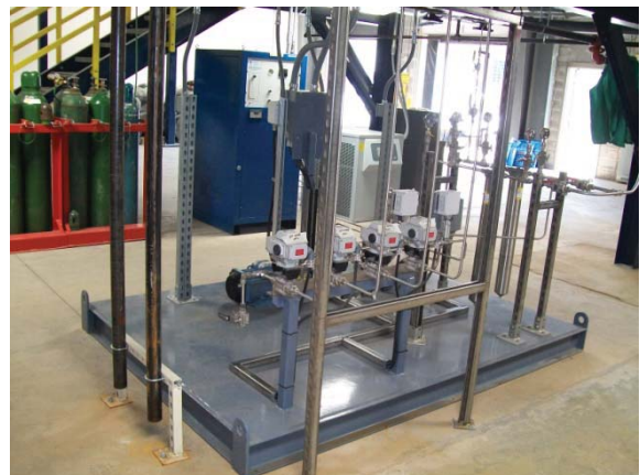
Figure 13: Two pump fogging skid.
