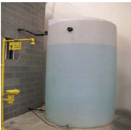
Figure 12: RO water storage tank.
